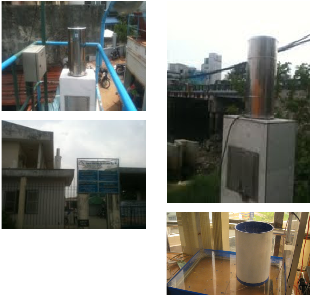
Fig 9. Installation of stations in Tan Qui Dong, Duong Quang Ham, Cau Bong and key laboratory DKS & KTHT.
