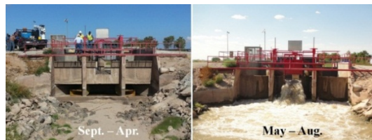
Figure 17. Installed units at Drop 8 Station
